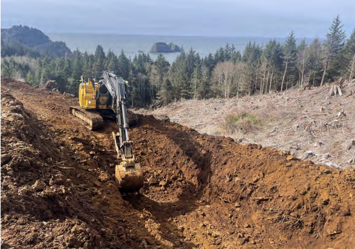
View of foundation excavation for MSE Wall No. 2 near the south project entrance on 03/27/23.
