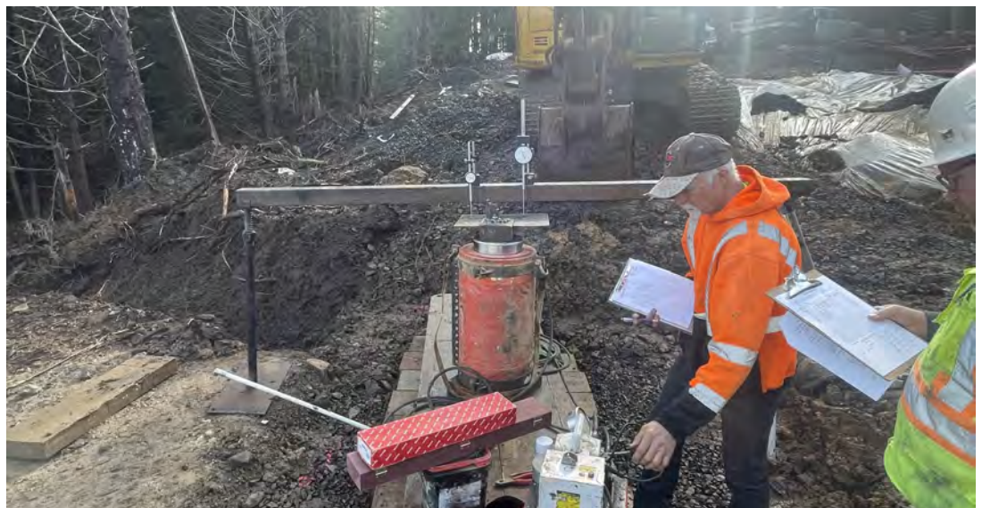
View of stress test on sacrificial ground anchor near proposed soldier pile wall on 03/29/23.
