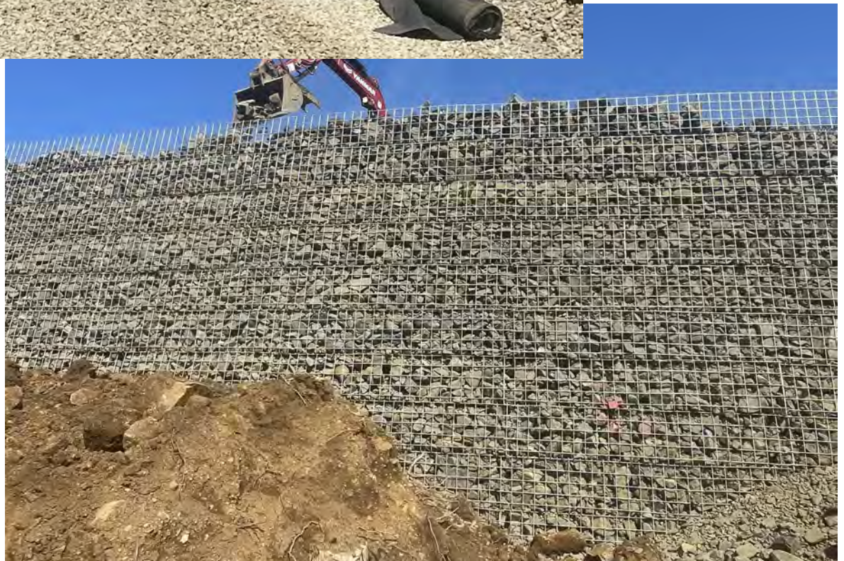
View of face rock placement on second to last course on MSE Wall No. 2.
