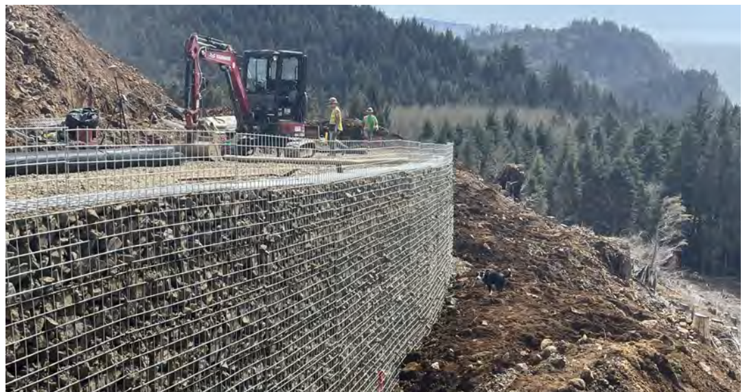
View of the beginning of the second to last course on MSE Wall No. 2.
