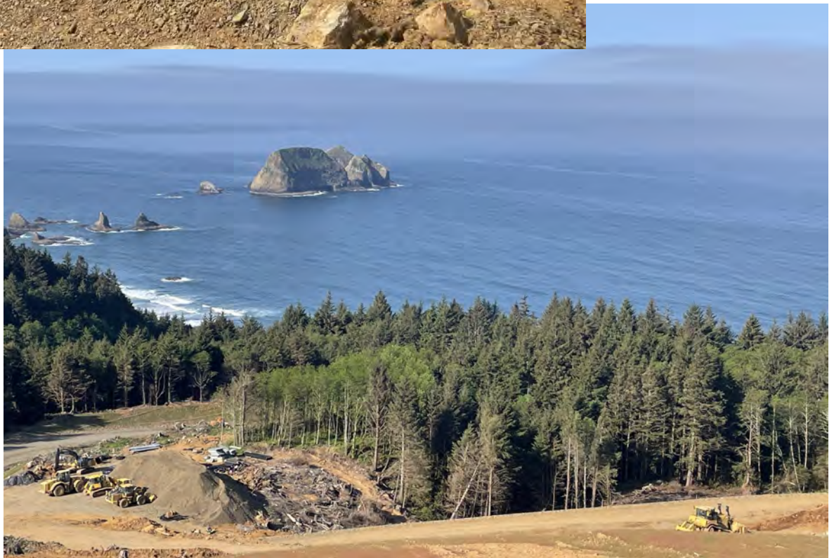
View of MSE Wall No. 3 after completion as seen from the top of the hill leading down to the wall.
