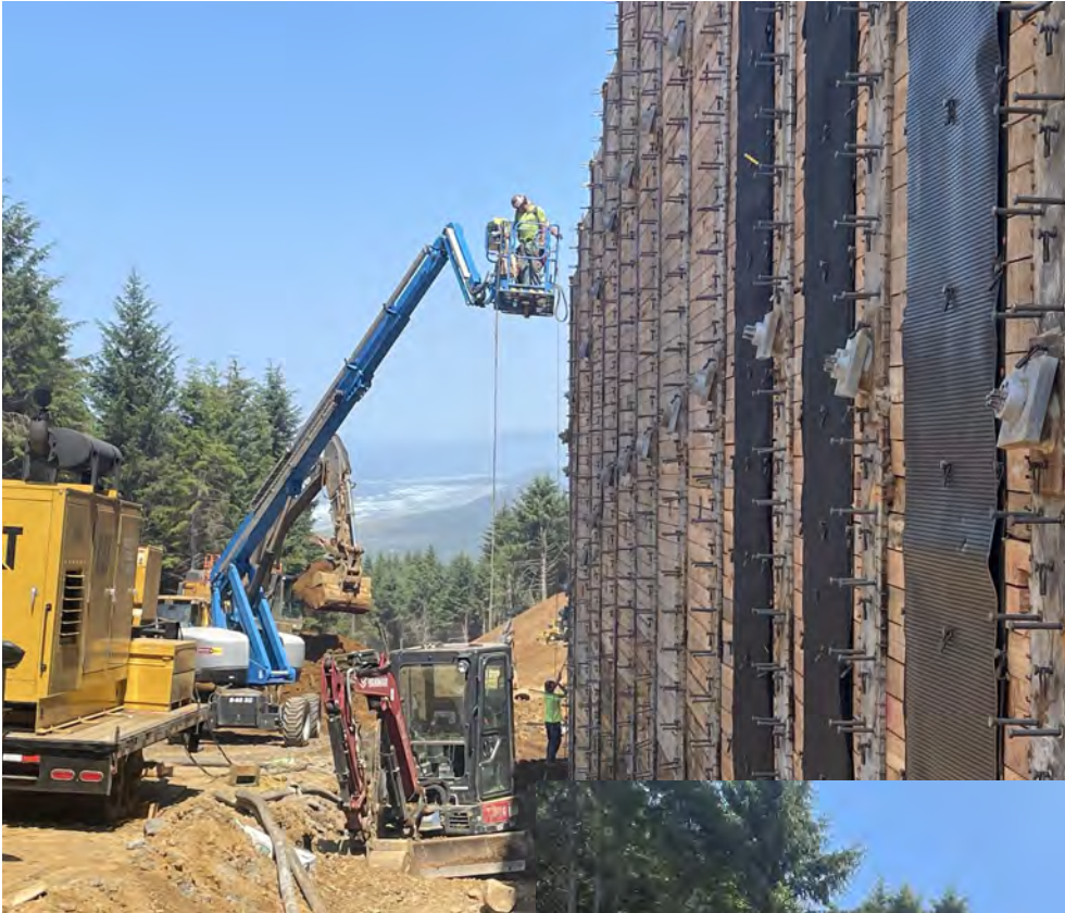
Alternate view of soldier pile wall showing headed shear stud welding and completed timber lagging installation.
