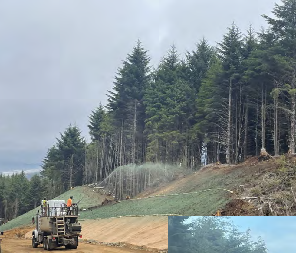
View of contractor spraying seed, fertilizer, and mulch from a hydroseeder on the north side of the project.
