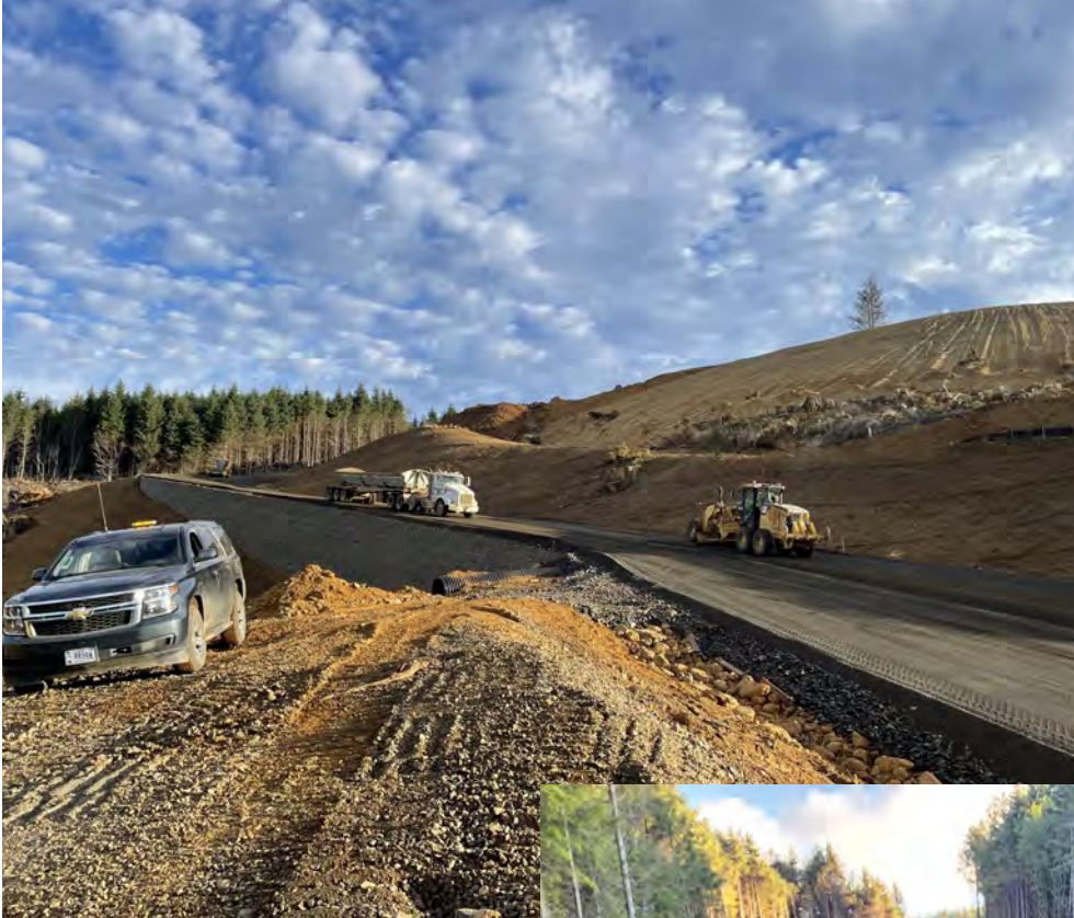
View of the contractor placing 301 Base Grade D aggregate for roadway base atop one of our MSE walls on the south side of the project.
