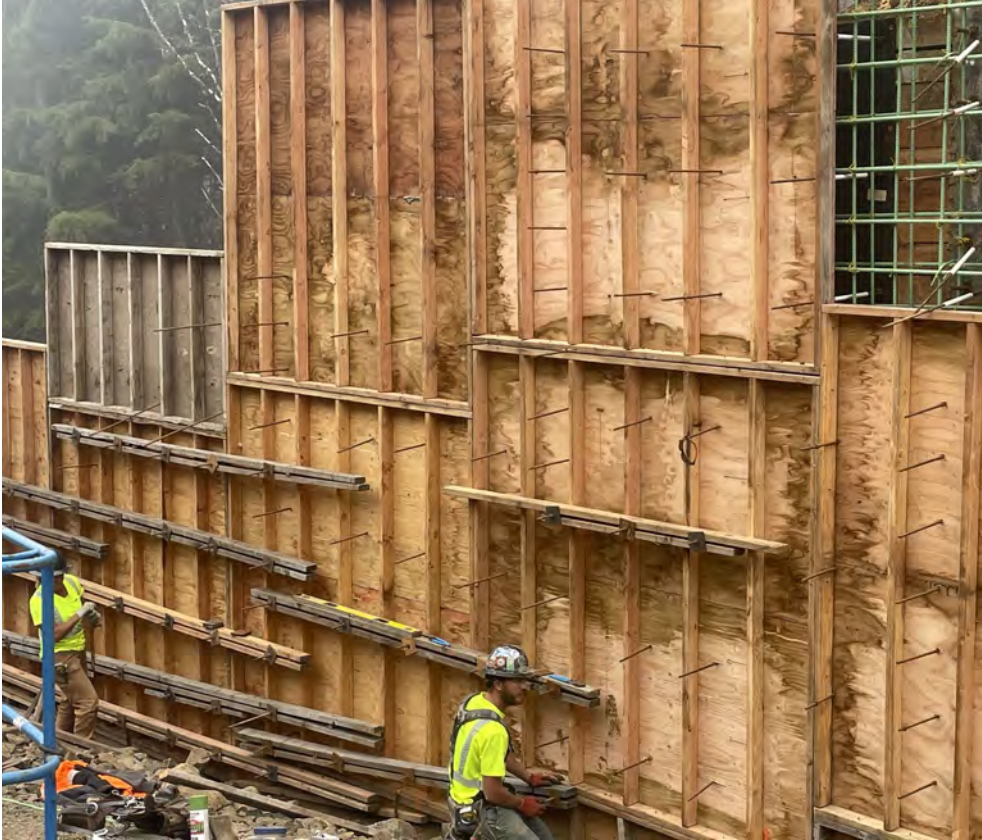
View of concrete form placement at the Soldier Pile Wall preparing for concrete placement on Friday.
