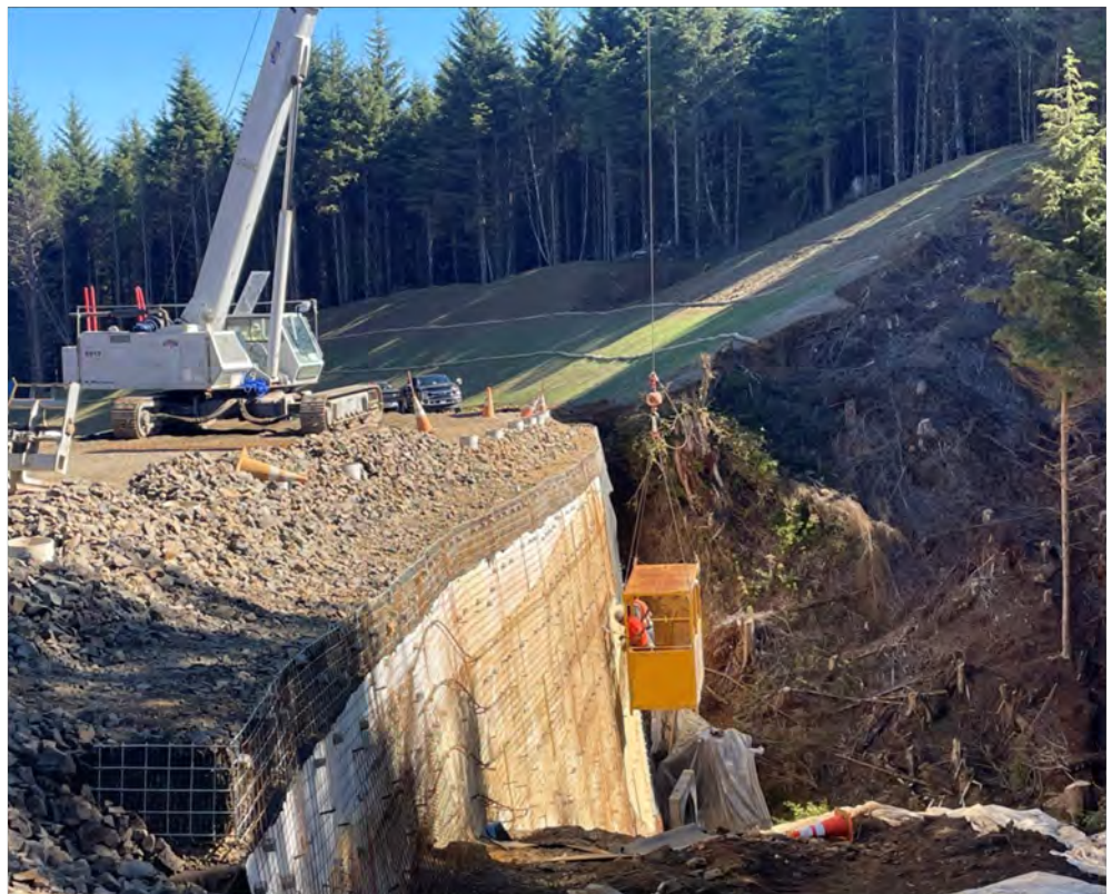
View of reinforcement installation on Geofoam Wall in preparation for continuing shotcrete placement beginning next week.
