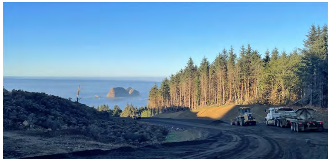
View of roadway aggregate placement near the south end of the project.
