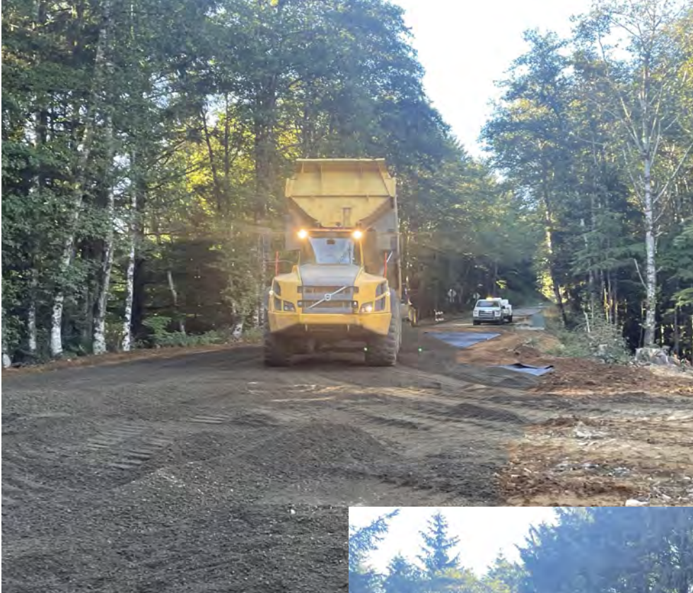
View of base aggregate placement on Cape Meares Loop near the south entry of the project.
