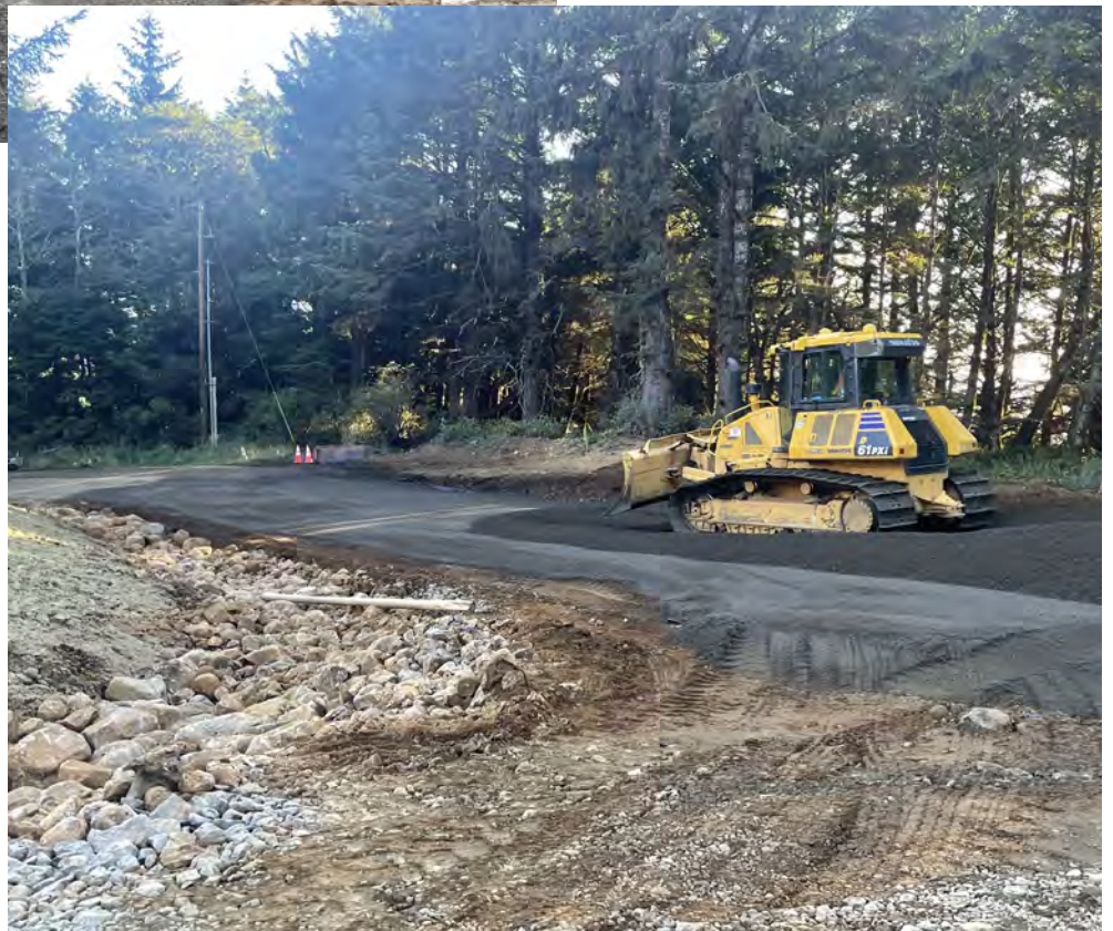
Alternate view of base aggregate placement on Cape Meares Loop near the south entry of project.
