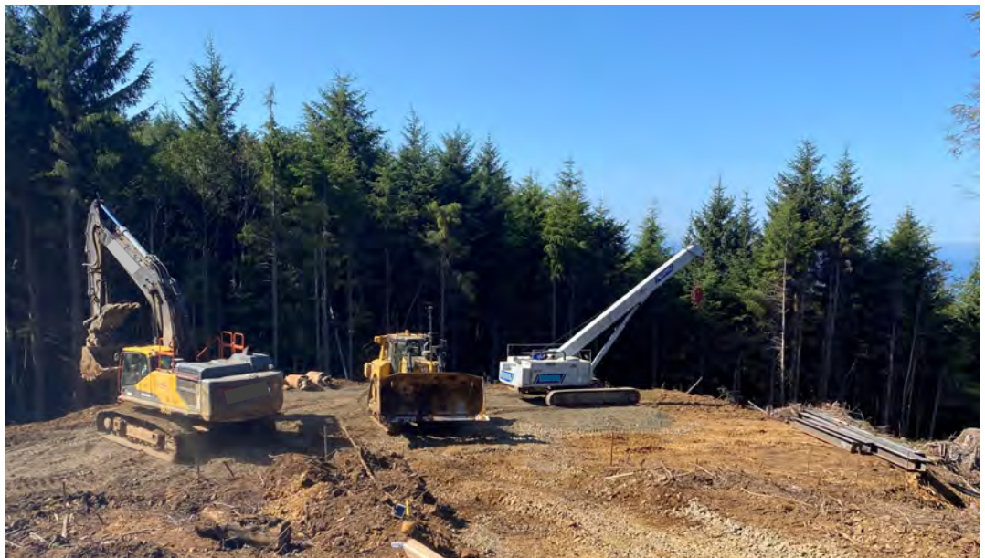
Setting up equipment to drill and set piles on the North side
