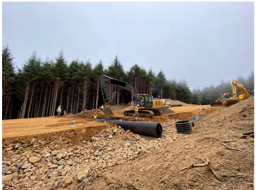
Setting and backfilling an HDPE pipe to ensure proper drainage of the roadway
