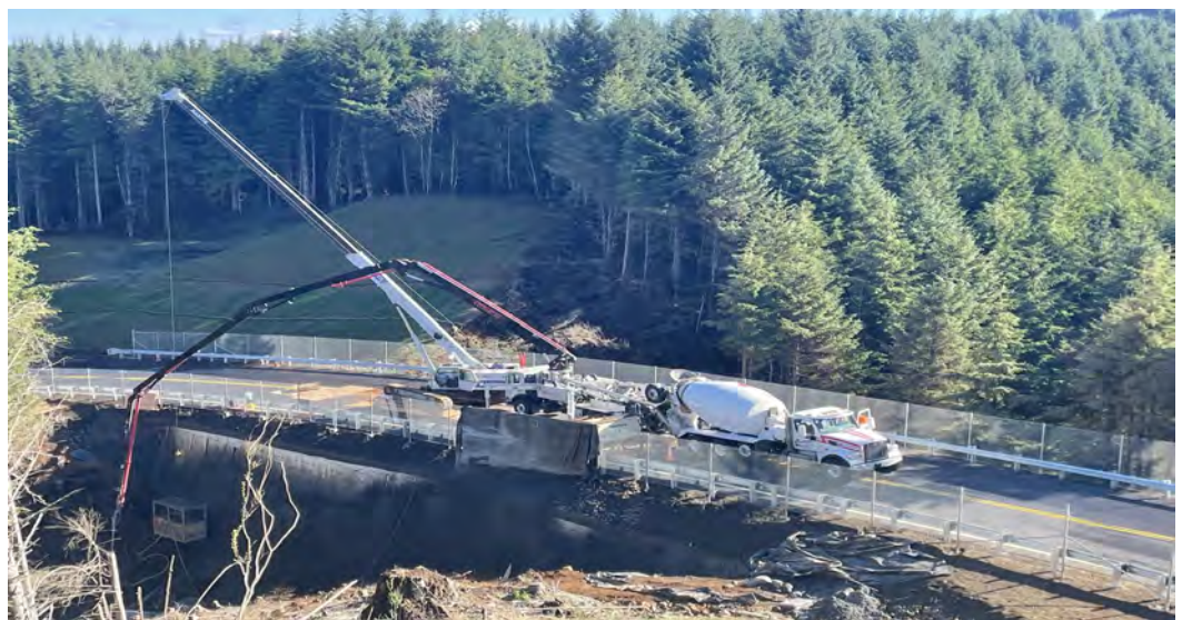
View of workers supported by crane to apply shotcrete on geofoam wall.
