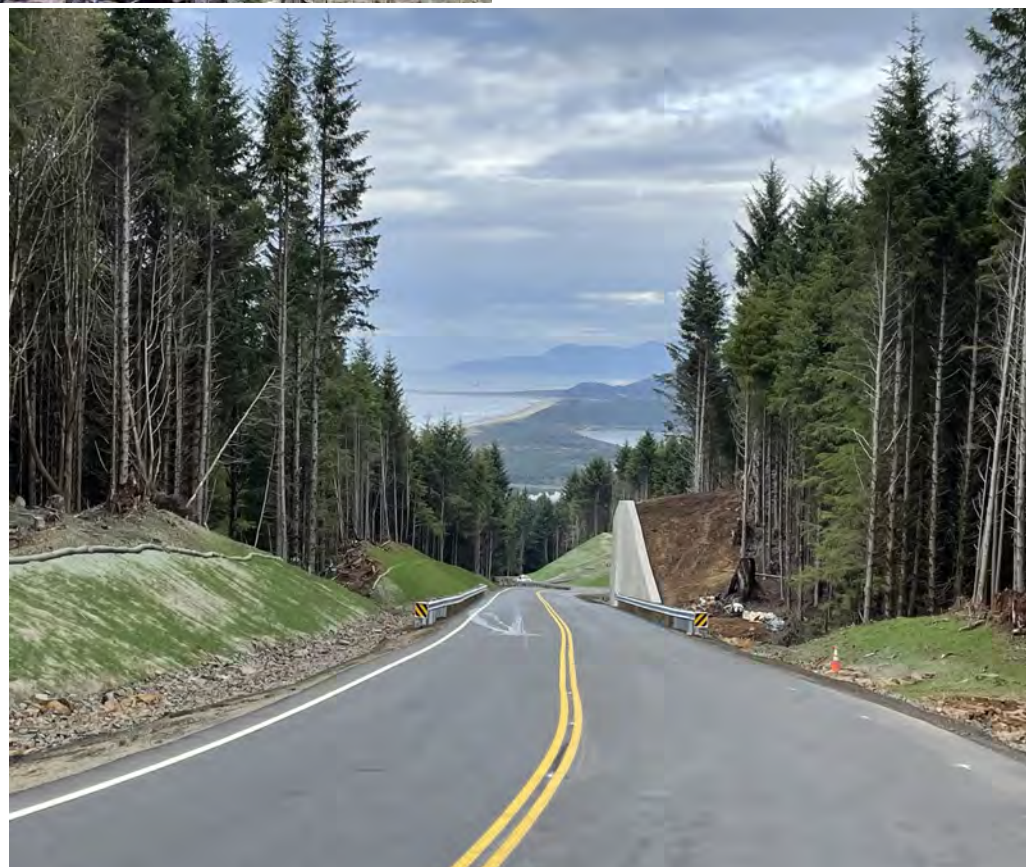
View of north end of project stream 5 area gate guardrails and soldier pile retaining wall.
